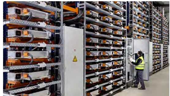
Figure 4.5: Second-Life Energy Storage Application for BMW Electric Vehicle Batteries
