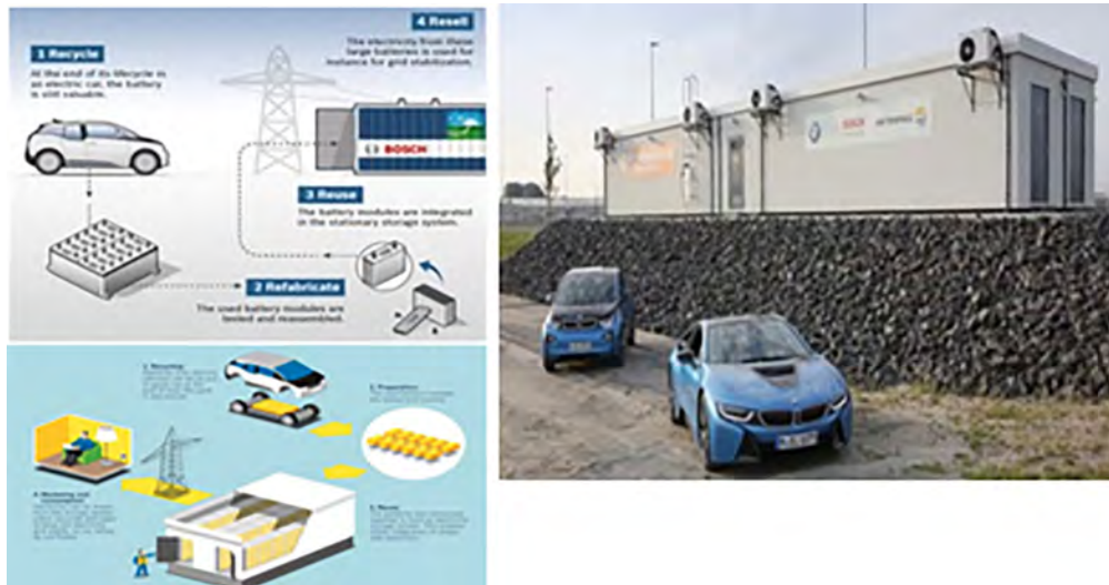
Figure 4.6: BMW–Bosch Second-Life Electric Vehicle Battery Demonstration Project
