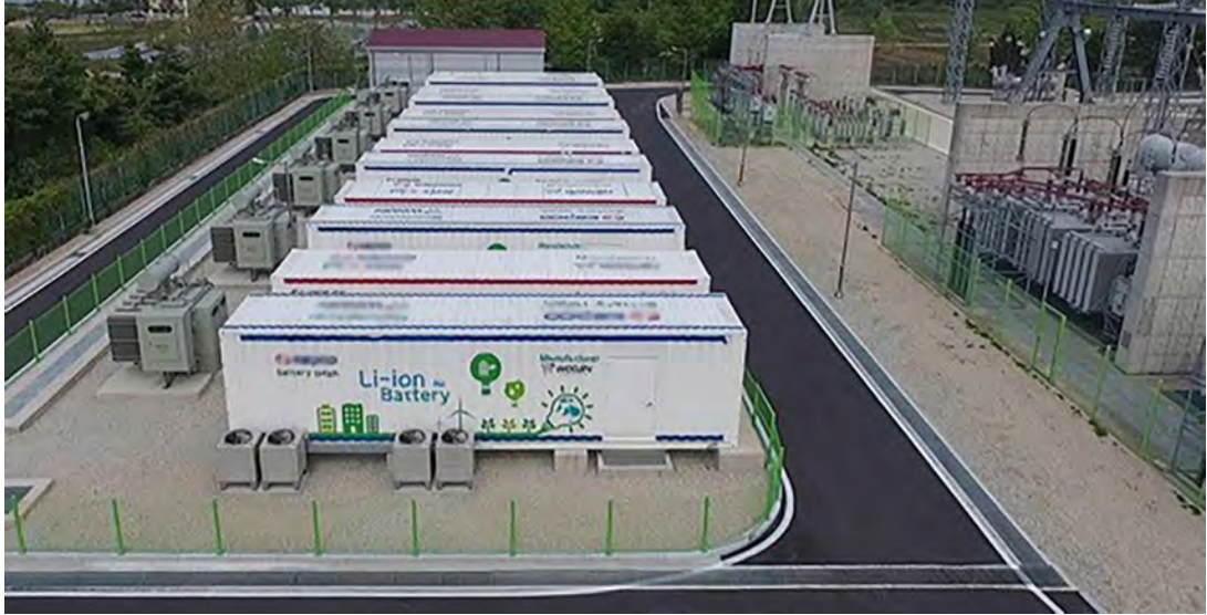
Figure D.4: Sokcho Battery Energy Storage System
