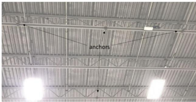
Fig. 8. Ceiling deployment 7.2 m above ground using POE daisy chained anchors
