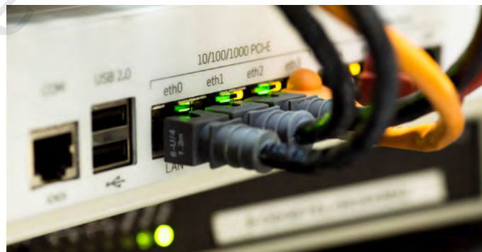
Figure 10.12: Cables connected to a network switch
